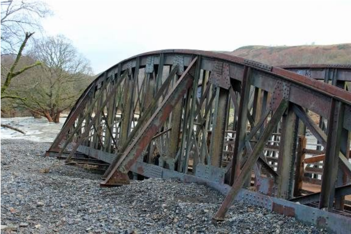
Brundholme Bridge now beached. Photo by Fred Lawton.
